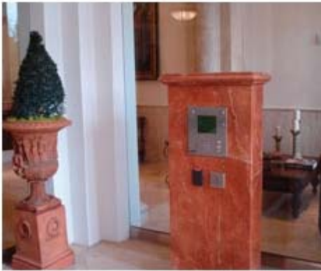
HID Global's ProxPro wall switch proximity readers provide access control for about 50 doors throughout the Veranda Park development, plus a telephone entry system by DoorKing provides further access control protection for the residential areas.
