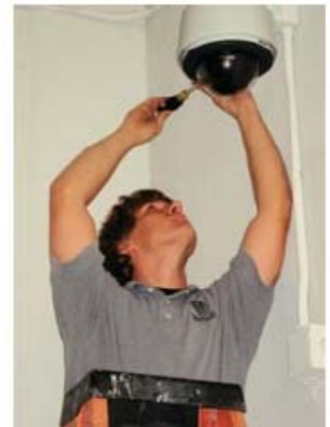
The more than 100 cameras installed by SmartWatch Security & Sound throughout the Veranda Park project include a combination of Pelco's Spectra IV p/t/z model, and ICS150 and ICS110 Series fixed domes. The cameras operate on an Endura IP-based video surveillance system.
